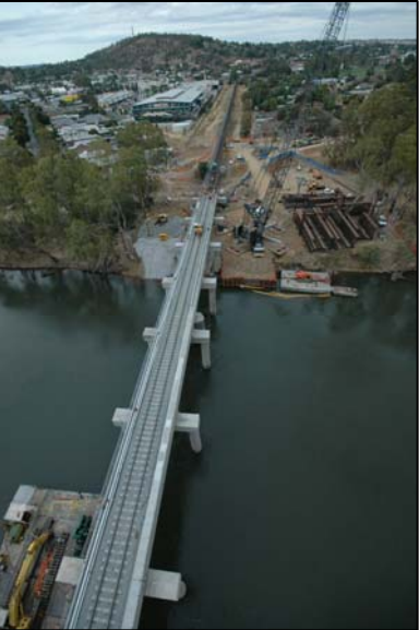
Rail Bridge over Murrumbidgee River, Wagga Wagga, NSW Reproduced with permission of Arenco, Construction Contractor for the project.
