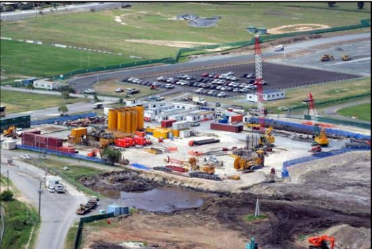
Gold Coast Desalination Plant, Gold Coast, Qld
